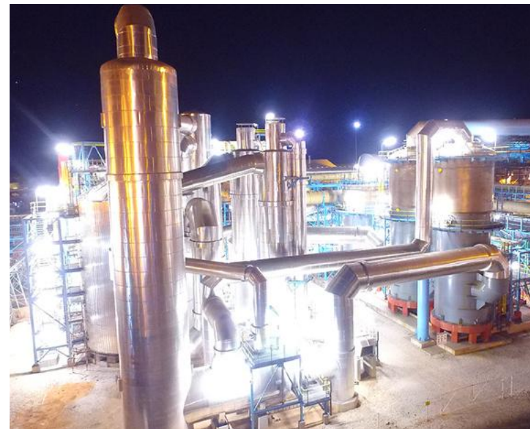
Tsumeb Smelter 烟气制酸设施
